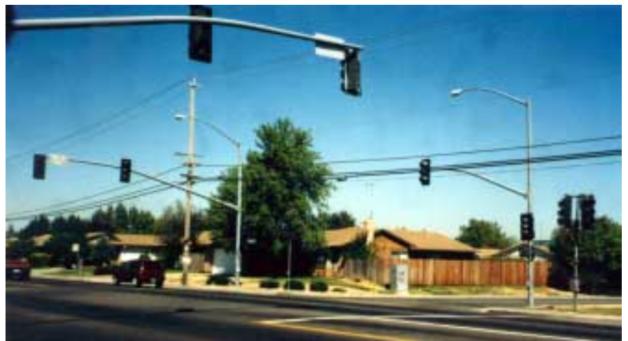
New traffic signals at Elder Creek and Sunrise South Drive/Cougar Drive. New signals are planned for a number of other key intersections throughout the City.
