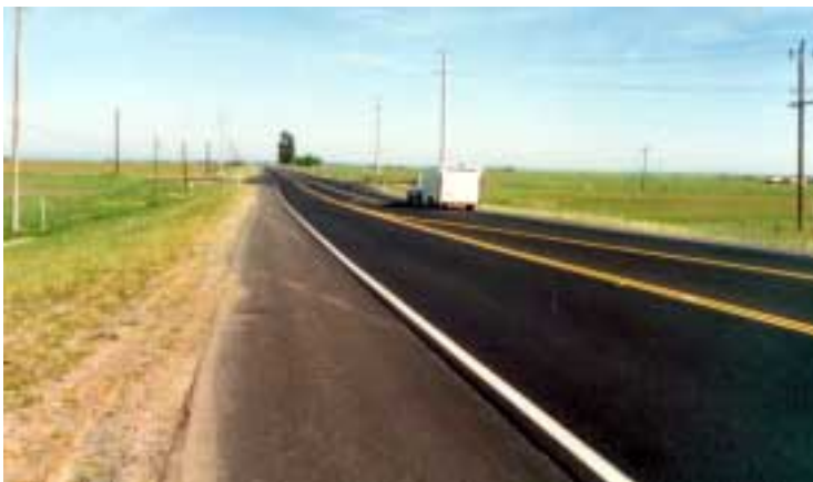
New safety shoulders on State Route 16 (part of the Jackson Road widening project between Tree View Road and Rancho Murieta)
